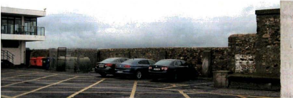
Figure 27: Area of wall to be removed to north of the former Harbour Master's House
